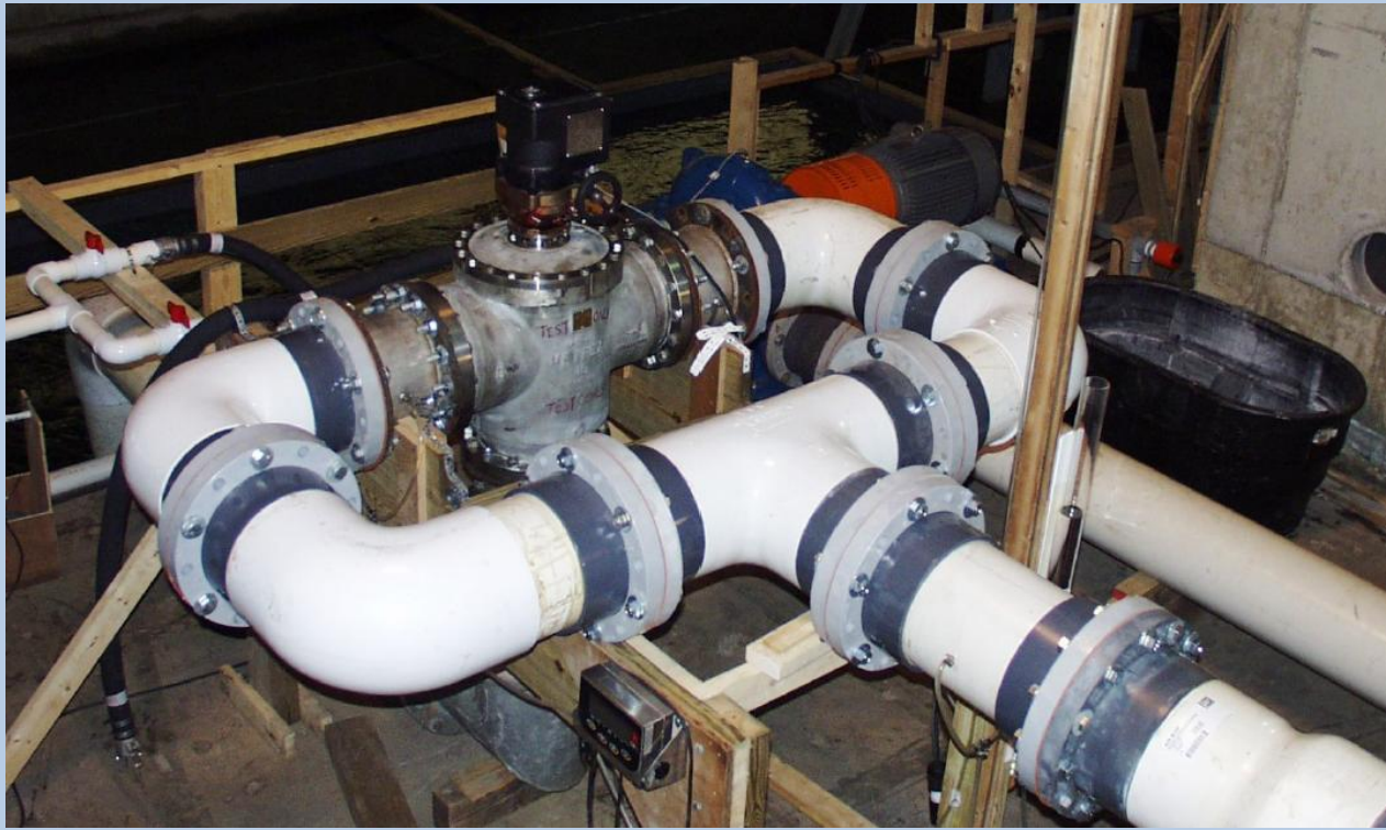
Figure 4- Metrex 3-way valve in the endurance test loop
